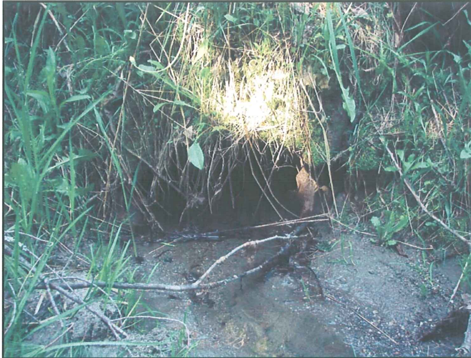
Photograph 1: C-03 (Inlet) – Excessive Sediment Obstruction
